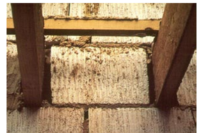
Timber joists built into a block wall - a poor detail for airtightness. Far better to use joist hangers and avoid the problem. Source: P. Warm.
