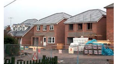
New houses tend to suffer in particular from timber floors and dry lining, service ducts and areas of unplastered blockwork, along with simple shrinkage cracks associated with the initial drying out period. Source: www.dilwyn.org.uk.
