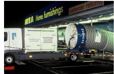
An example of a very large fan being used to test an Ikea Store. Source: HRS Services Ltd. www.air-tightness.co.uk
