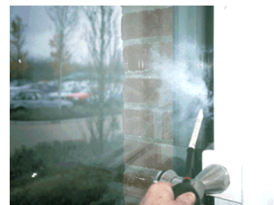
A smoke tracer allows for a view of the air leakage around the edge of this window frame while the building is depressurised. Source: A. Leaman & W. Bordass, www.usablebuildings.co.uk
