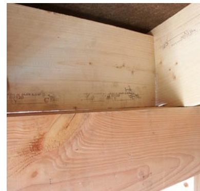
Some forms of construction cannot be reasonably expected to be airtight, so airtightness measures have to be 'designed in' from the start. Source: C. Morgan.
