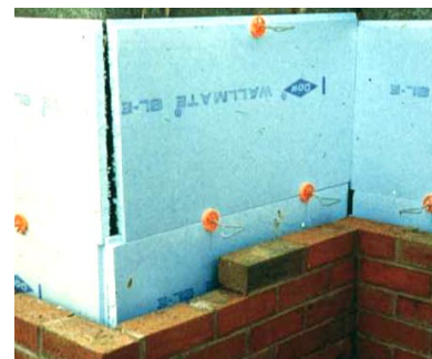
On the other hand, much work on site is unacceptable and so inspection and testing remain important ways to drive through better workmanship generally. Source: P. Warm.
