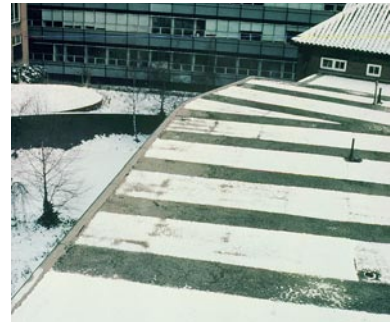
Snow melt on the roof of the Sheffield University Student Union Building showing the effects both of thermal bridging and (warm) air leakage. Source: Prof. R. Lowe.
