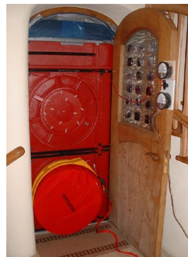
An example of a door fan within a panel affixed to the main entrance door of a new built house. Source: P. Jennings.
