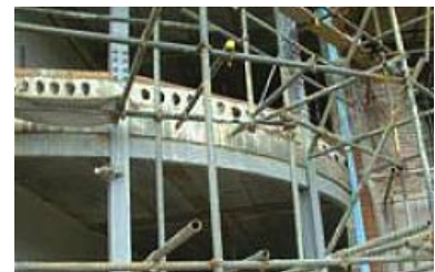
Concrete planks are not free of problems either. here, hollow planks have been left ungrouted where they meet the external wall, which could lead to extensive air leakage internally. Source: P. Jennings.
