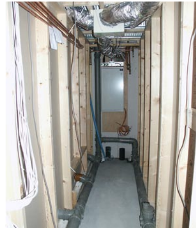
Services Zones or Rooms enable a range of services to be collected together before exiting the building, allowing most of the penetrations in the external fabric to be grouped and sealed effectively. Source: C. Morgan
