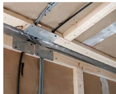
Service voids enable cables and pipe-work to be installed and altered without needing to penetrate the air barrier. Note however that if they are not run in conduit, protection may be needed against subsequent fixings. Source: C. Morgan
