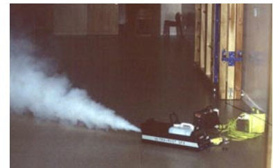
With a building pressurised, smoke can be let off to see if there are any leaks... Source: HRS Services Ltd. www.air-tightness.co.uk
