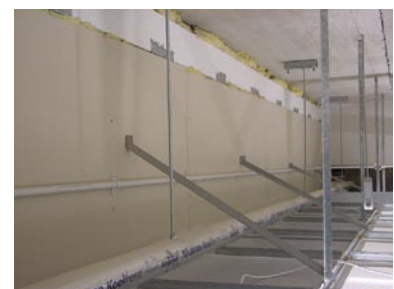
Above the suspended ceiling, the plasterboard is not continuous nor sealed, and mineral wool has been used which is not in itself airtight. Source: A. Leaman & W. Bordass, www.usablebuildings.co.uk
