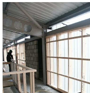
Buildings usually comprise a number of different components, creating a myriad of routes through which air can escape if not carefully sealed at each and every junction. The Designer's role is to simplify these details to reduce difficulties on site. Source: C. Morgan
