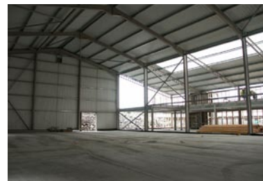
Air leakage measurements for large single storey buildings with non-exposed floors like the one above are more noticeably different because one of the previous expressions of airtightness excluded non-exposed floors from the measurement. Source: C. Morgan
