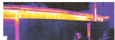
A thermographic image of heat loss through a Sports Centre, indicating a couple of potential air leakage sites. Source: P. Jennings.
