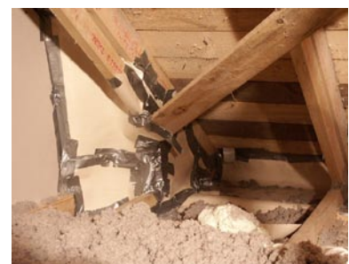
If not designed to be airtight in the first place, ad hoc solutions on site are not likely to be durable - or elegant! Source: C. Morgan
