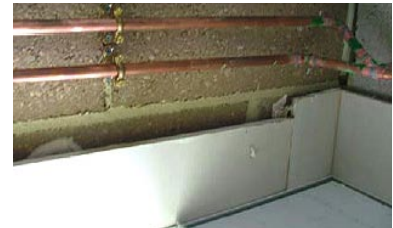
In addition to the intrinsic lack of airtightness, a problem of drylining is that it can create hidden pathways for air, as above, into the void above suspended ceilings and elsewhere throughout the building. Source: P. Jennings.
