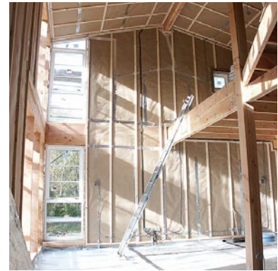
This building is almost ready for its first test. The vapour check is complete and accessible, before the plasterboard is fixed over, all windows and doors are in, but note that the gaps around the windows have yet to be sealed. Source: C. Morgan.
