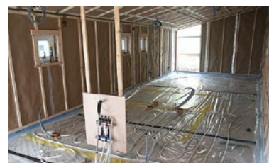
Buildings using slow response heating systems such as storage heating or underfloor heating can be vulnerable to discomfort caused by air leakage during certain weather conditions if they are not well insulated and carefully sealed. Source: C. Morgan.
