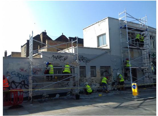
fig 28. The old bank building on day one of restoration, the dire state of the building before can clearly be seen from the layers of Graffiti and falling paint.
